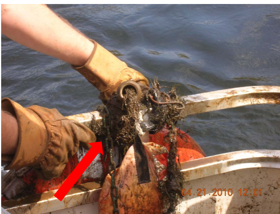
Lost intake screen and clogged with mud and vegetation
