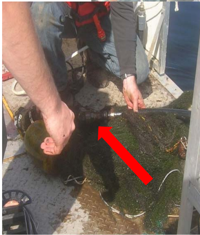
TID Intake #1 covered with weeds and mud
