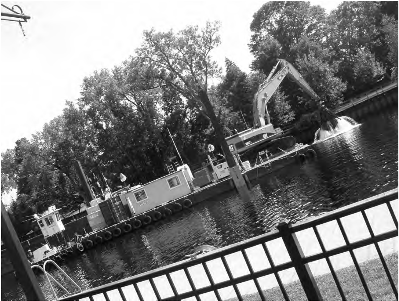
Figure 3. Dredge buckets should close completely before lifting their sediment load, but they leak excessively because obstructions prevent complete closure. Hudson River dredging site, July 28, 2009.
