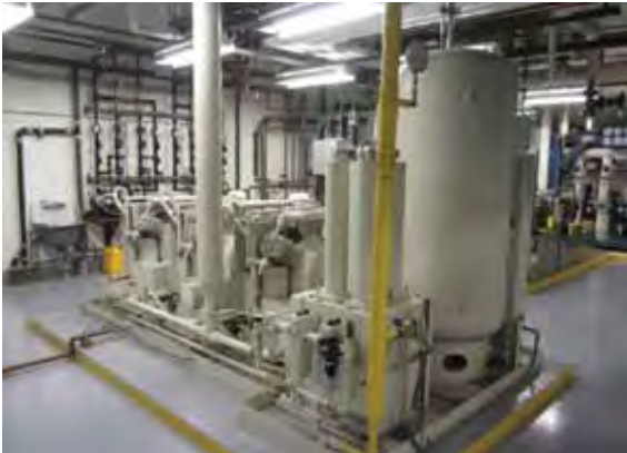
Medical air compressors
