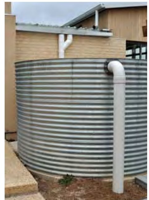
Rainwater collection system
