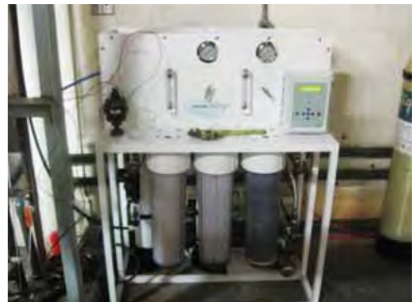
Reverse osmosis system
