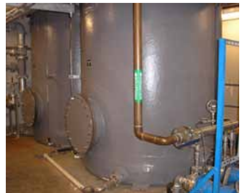
Two 2,500-gallon tanks storing air handler condensate and harvested rainwater for irrigation
