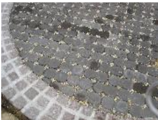
Figure 9 – Typical porous asphalt (top) and permeable paver (bottom) applications (Source: Philadelphia Water Department, 2012)
