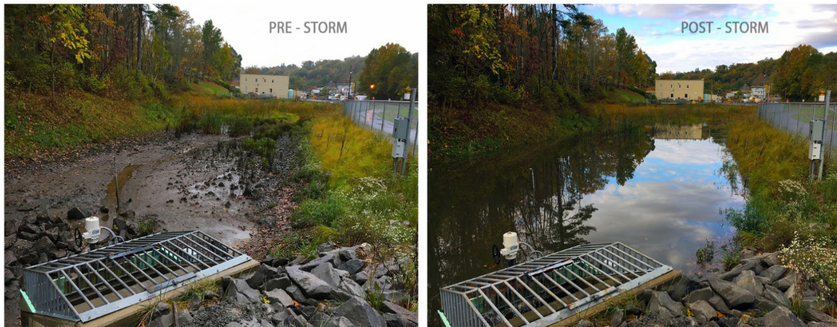
Figure 1. Pre- and post-storm conditions at the Ewart Avenue stormwater pond.
